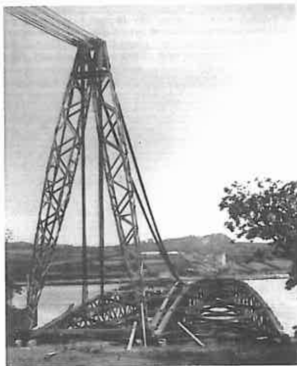
fig. 6 – 2.06.1926. Levage des bigues servant au soutien du câble transbordeur côté Plougastel. 2.06.1926. Lifting of demicks serving as a support for the trussing cable on the Plougastel side.
